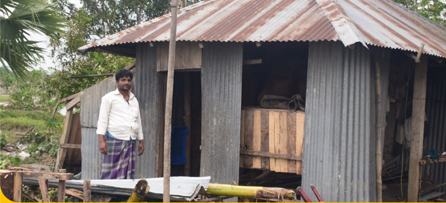
Halim is standing in front of his house at Southkhali Union, which is damaged due to Cyclone Amphan.
